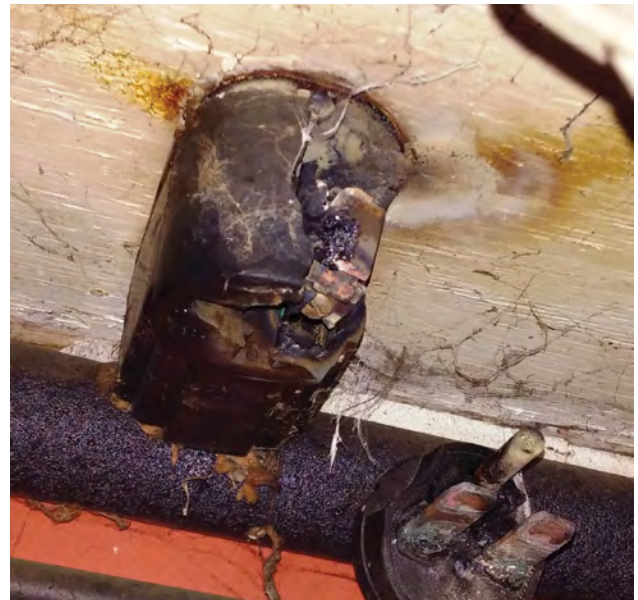
Picture 14: Receptacle damaged from corrosion and arcing
