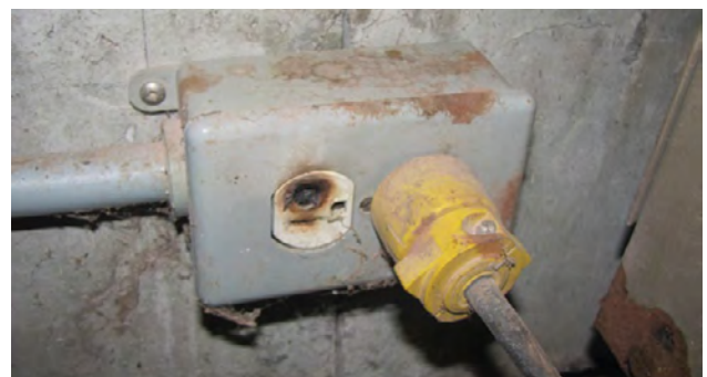
Picture 9: A receptacle with a burnt terminal
