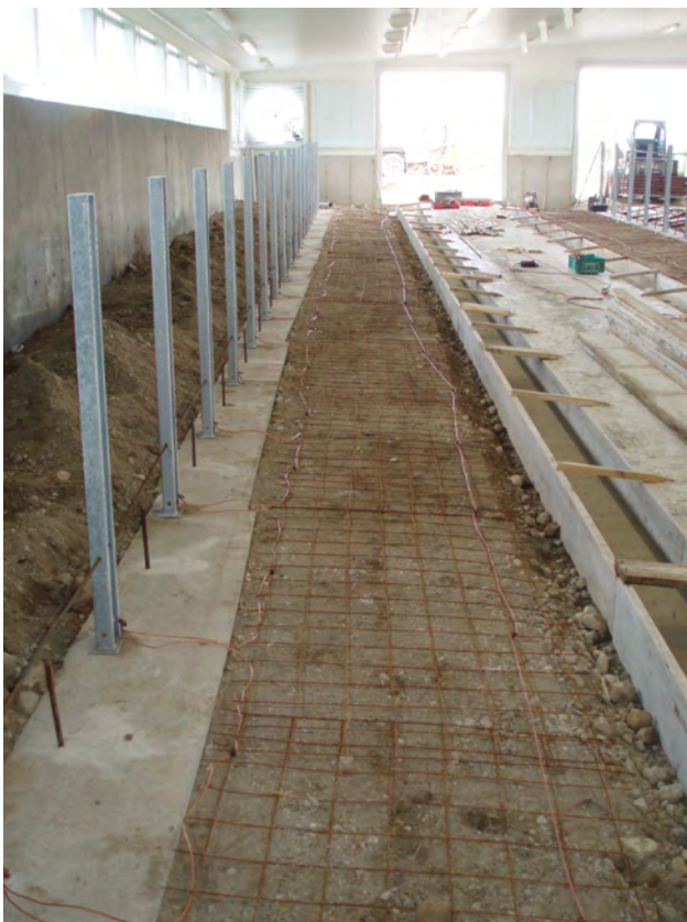
Picture 3: Bonding conductors attached to the metallic mesh prior to pouring concrete creating a equipotential plane
