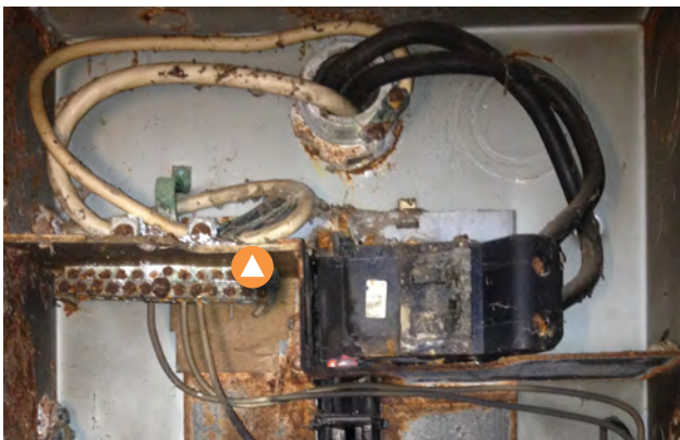
Picture 7: Electrical panel showing signs of corrosion
