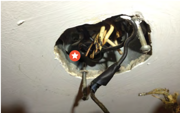
Picture 6: Conductors missing connectors in an outlet box.
