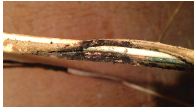
Picture 4: Damaged outer jacket of cable
