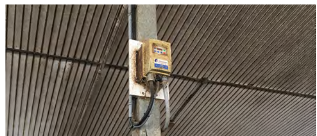
Picture 15: Variable Frequency Drives installed on a column
