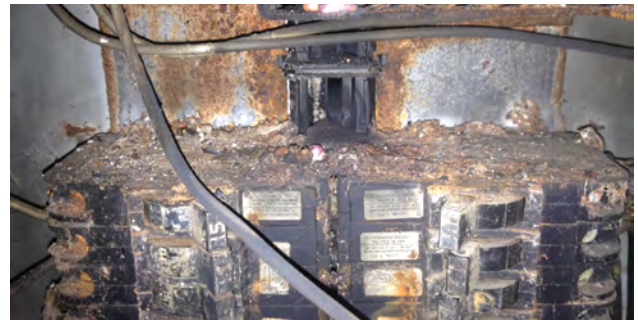
Picture 8: An electrical panel with signs of corrosion
