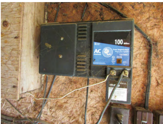
Picture 16: Power supply for an electrical fence
