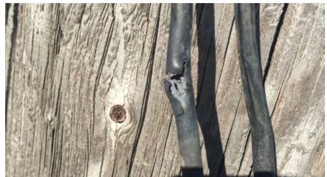
Picture 2: Damaged ground conductor
