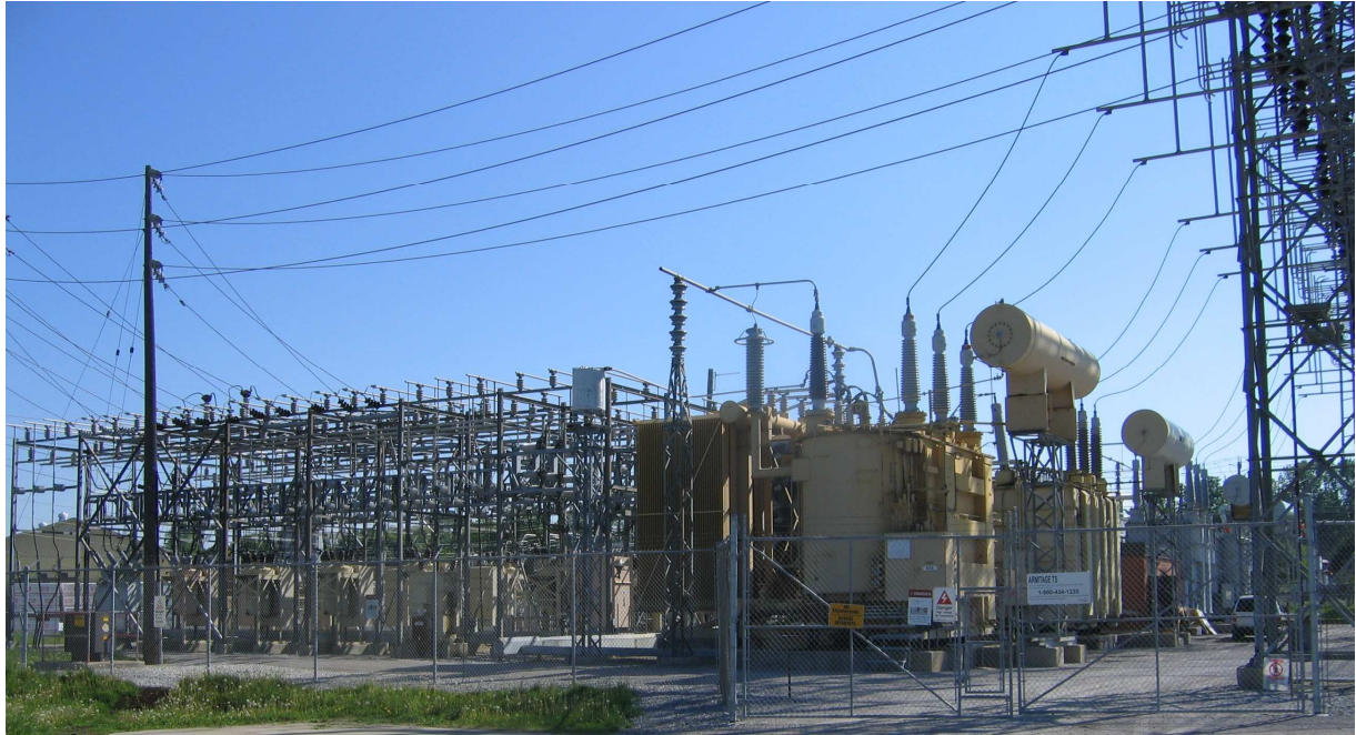
Figure 3-1: Armitage Transformer Station
